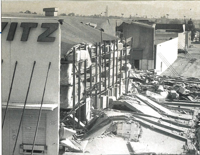
The back wall of this store collapsed.
