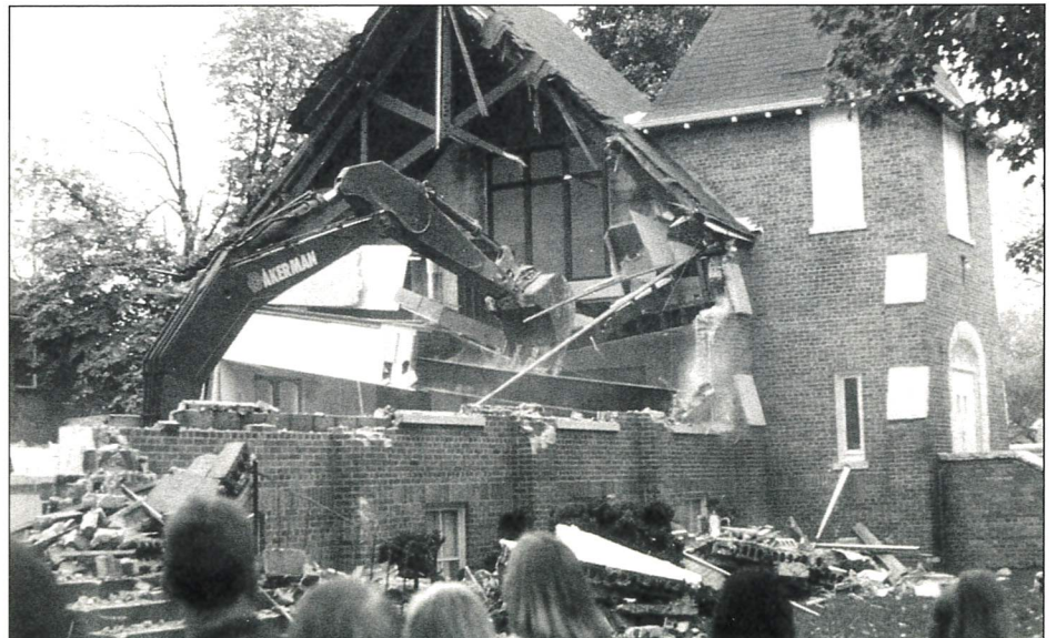
Atonement, Milwaukee, razed their original church and school, built in 1931, to make way for a new school. Construction on the new building began in November. Atonement rented facilities this year for their school.
