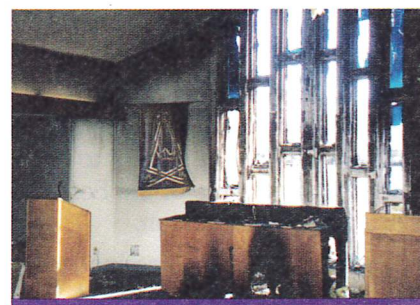
The arsonist broke this stained glass window in order to pour in the gasoline and throw the match.
