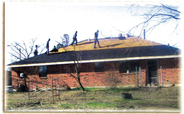
A Builders For Christ team works to put a new roof on the parsonage at Crown of Life, New Orleans, La.
