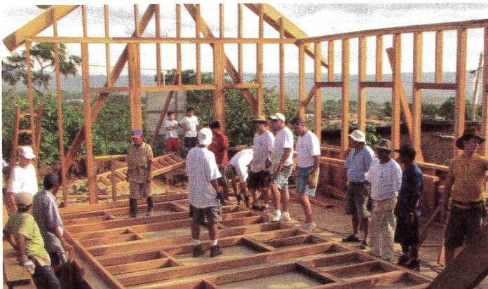
Members of Living Word, Waukesha, Wis., help build a church in Tarapoto, Peru. "One of the best things was going halfway across the world and finding brothers and sisters in Christ," says John Borgwardt, pastor at Living Word.
